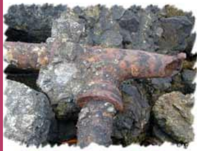
THESE PIPES ARE IN THE MIDDLE OF CHEMICAL CHANGES AS THEY RUST.
